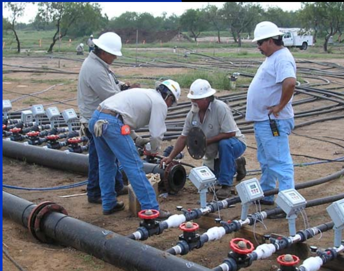
Wellfield piping and instrumentation. (below)
